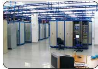
IDC engine room
